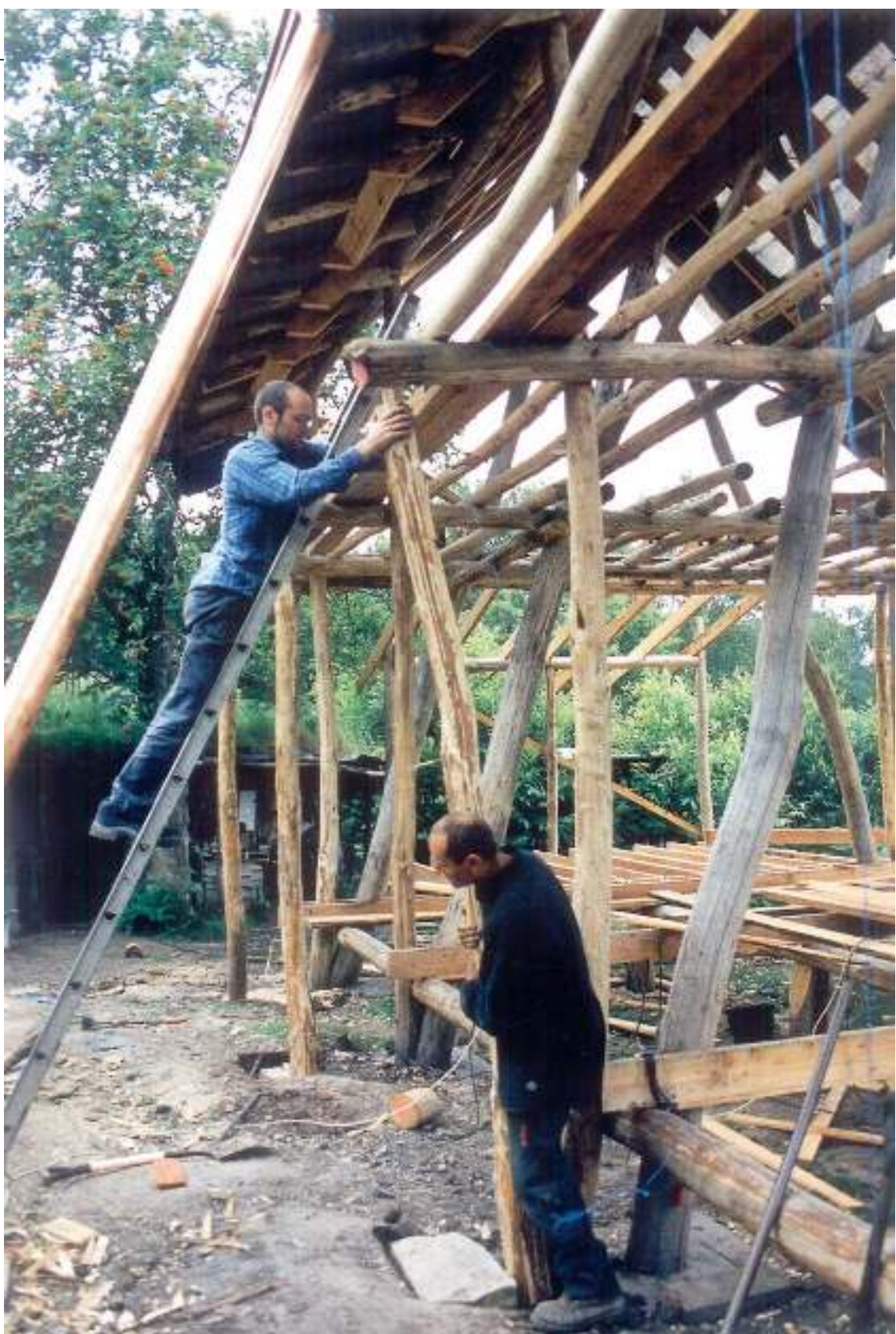
We have also promoted craftsmanship in a big way. (Cruck-Framed Woodland House) (© Ben Law)
